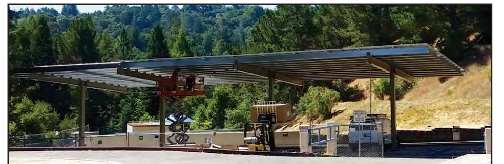
Solar panels at Glorietta Elementary School have been installed in two locations: the front parking lot and the upper parking lot.
