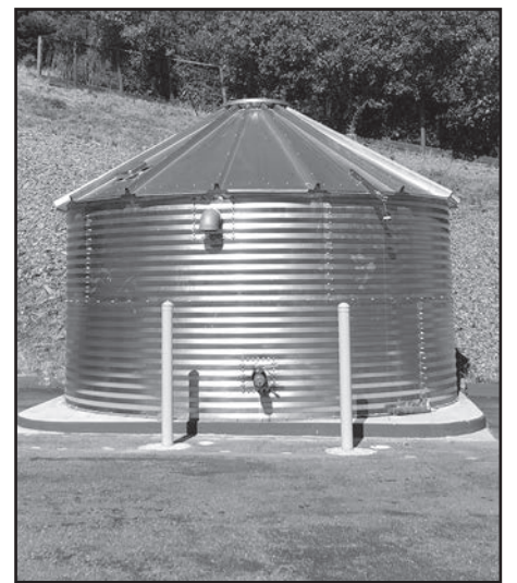
LYNN KALMAR Sleepy Hollow Elementary School's 10,000 gallon tank gives firefighters an immediate water source in case of wildfire.
