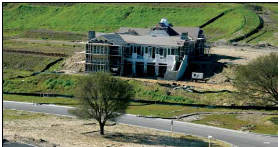
One of the homes on Rabble Drive currently under construction with one of the mature Oak trees uprooted during grading and then replanted throughout the housing development.
