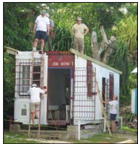
The Karplus clan had this steel container sent ahead and then added electrical wiring, shelving and more to make it into a library.
